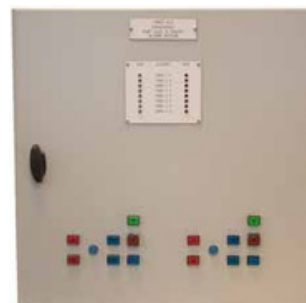
Cabinet with alarm overview on each tank
