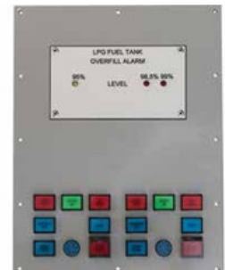
Panel with alarm overview on each tank
