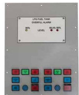
Panel with alarm overview on each tank
